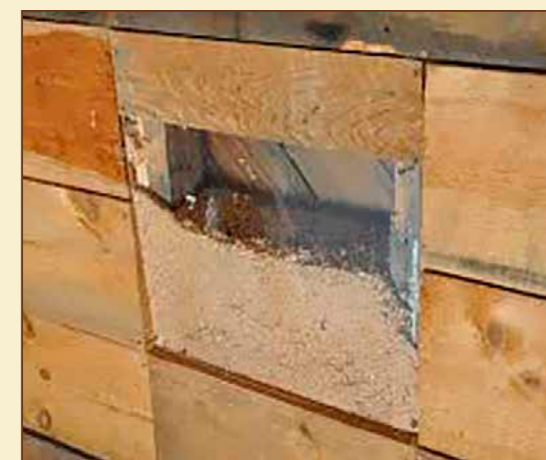
Cutaway view of an ice house wall, showing the sawdust fill typically used as insulation.
